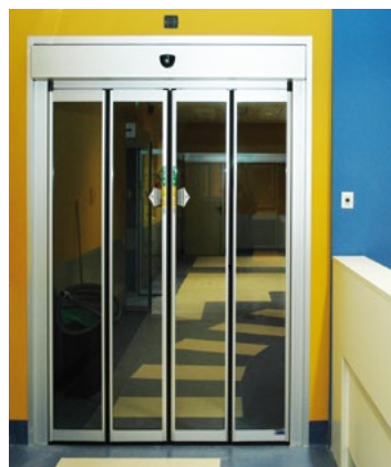
FDA filters, internal compartmentalization
