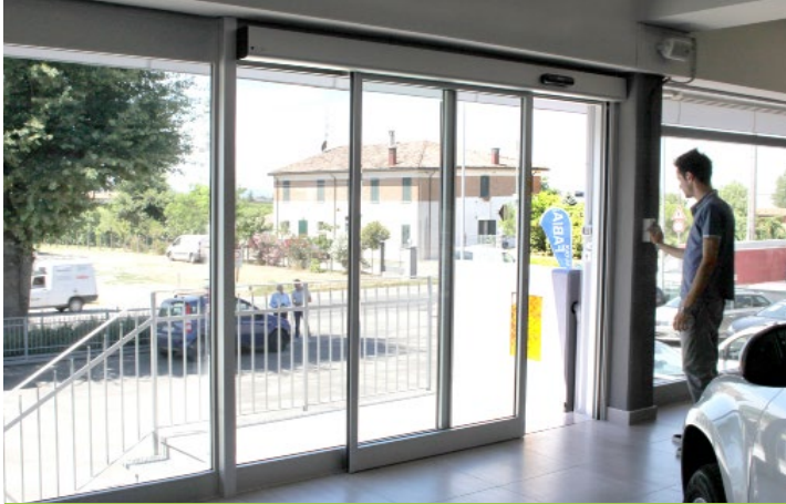
RID door actuation of the emergency button in dangerous situations
